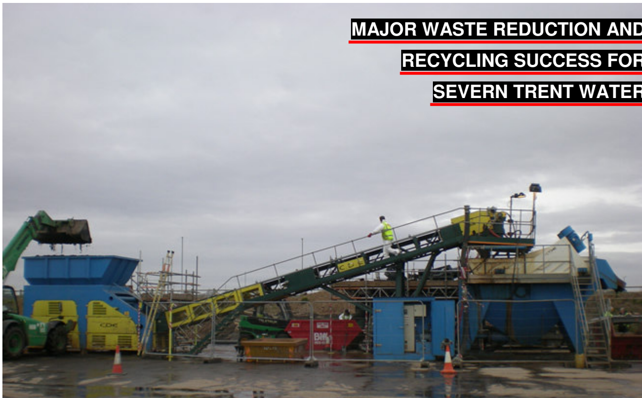
Dmax - portable plant installation at Minworth Sewage Treatment Works
