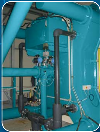
Filtrate Discharge Manifold
